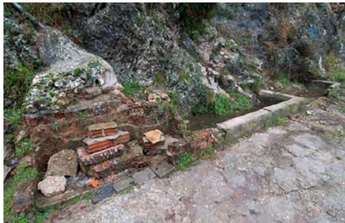
Fig. 4: Water trough before restoration. Photo: AHE.
