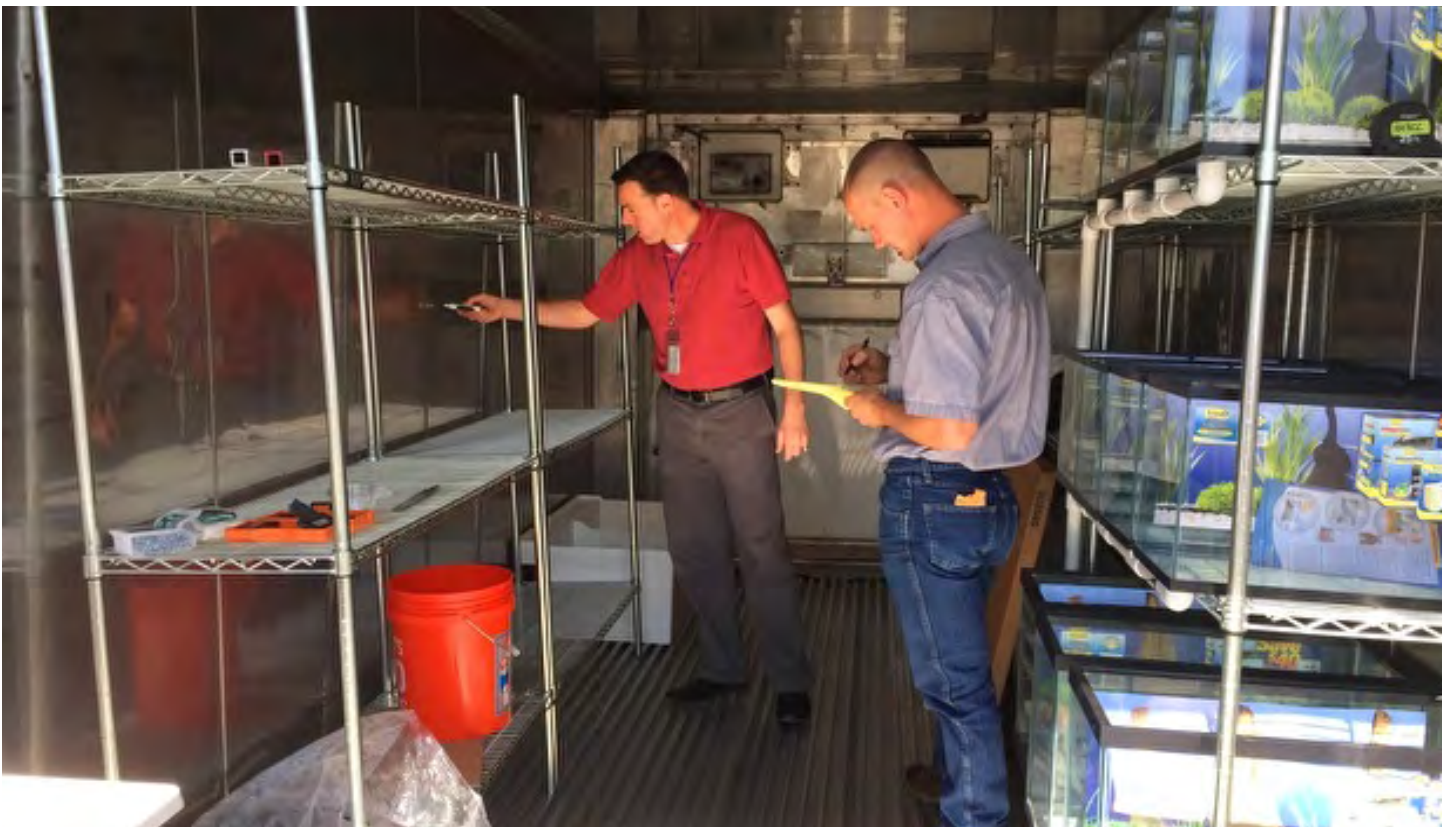
The containers are inspected by an electrician in preparation for hook-up to a power supply. Photo by: Brandon Greaves.
