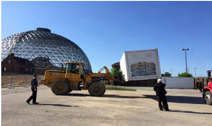
The shipping containers finally arrive at the Henry Doorly Zoo & Aquarium! Time to get to work! Photo by: Brandon Greaves.
